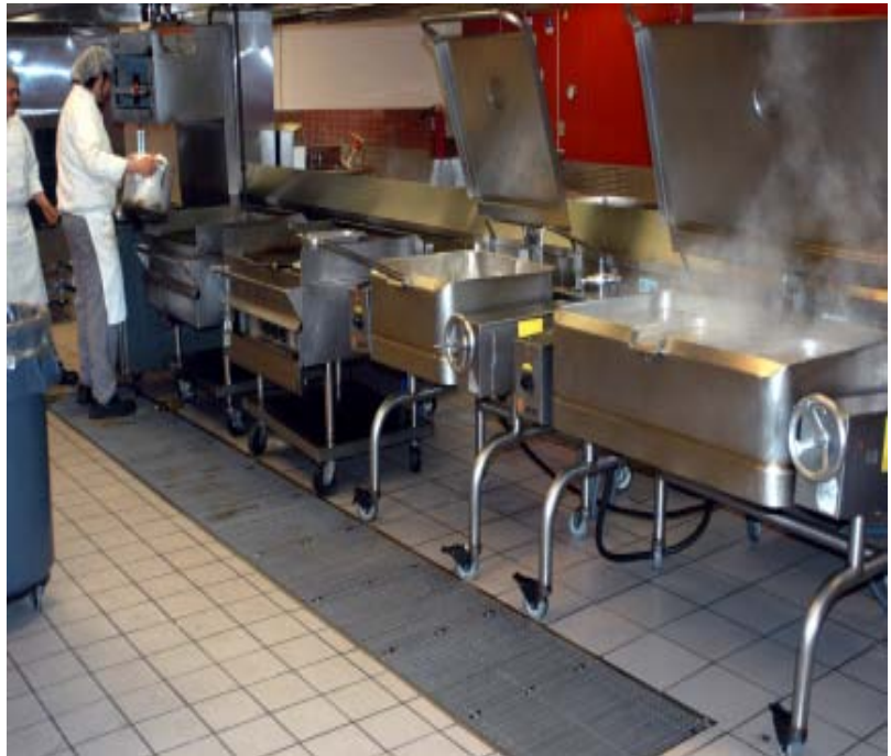
Hot Production Area (partial)
